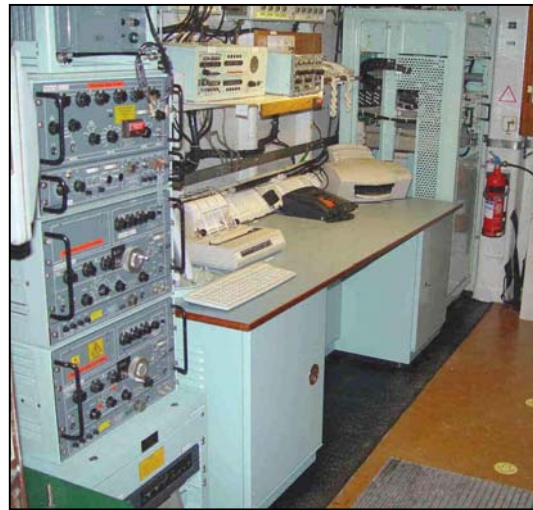
A FOUR-CUPBOARD UNIT INSTALLED IN A MCMV MAIN COMMUNICATIONS OFFICE
