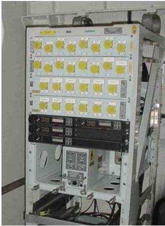
19" equipment rack, housing six and eight way patch panels
